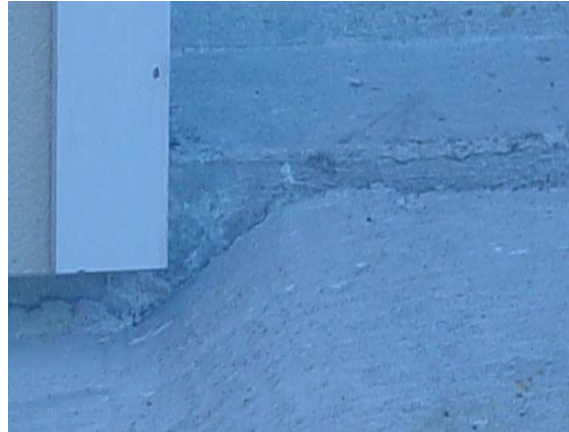
Photo depicts formed concrete at garage door to provide minimum 50mm level change (centre) and 50mm ground clearance below Hitex Diamond EIFS Cladding (left).
